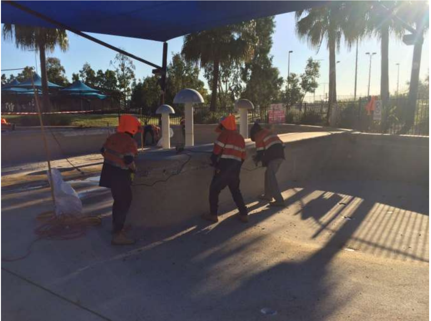
Leisure Pool - pebblecrete finish being removed to undertake repairs to 'drummy' surfaces
