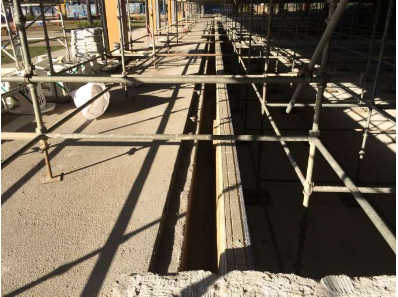
50m Pool (east side) - wet deck removed with hob tiles removed in the foreground
