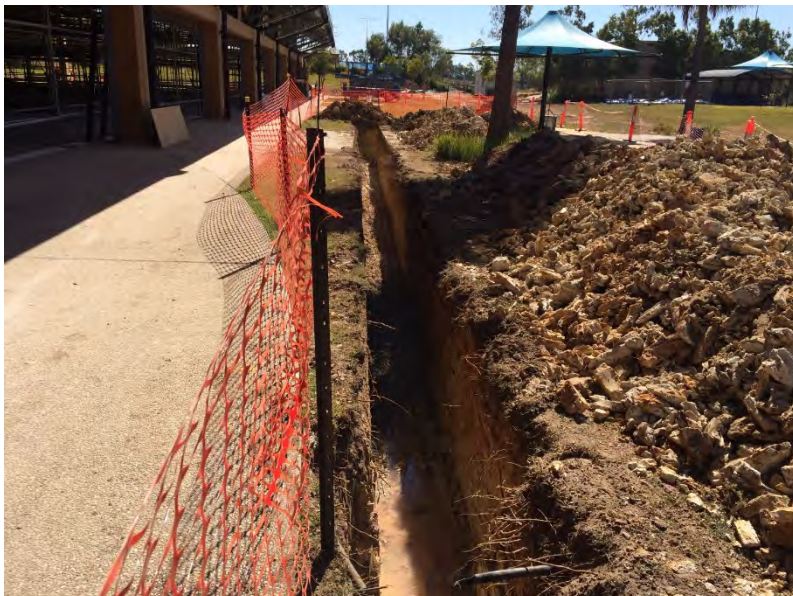
Excavation to the east face as part of the preparation to install the new 50m pool return water line
