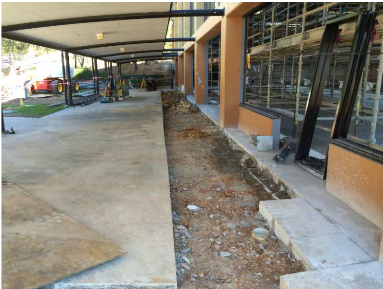
Paving removal in preparation for the excavation required to install the new 50m pool return water line
