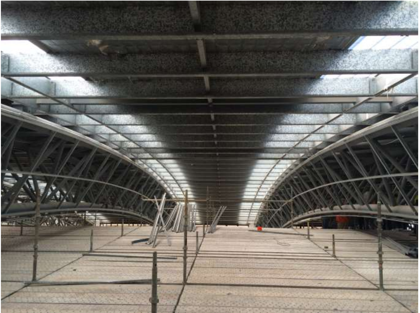
Roof structure in the early stages of being prepared for the installation of the new ceiling
