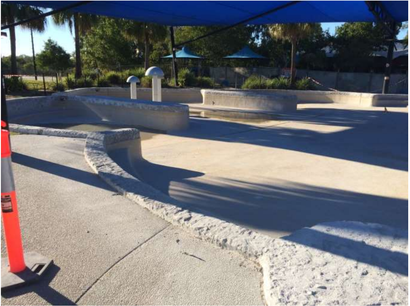
Leisure Pool - defective pebblecrete surface material removed with repairs and preparation for the new finish to follow
