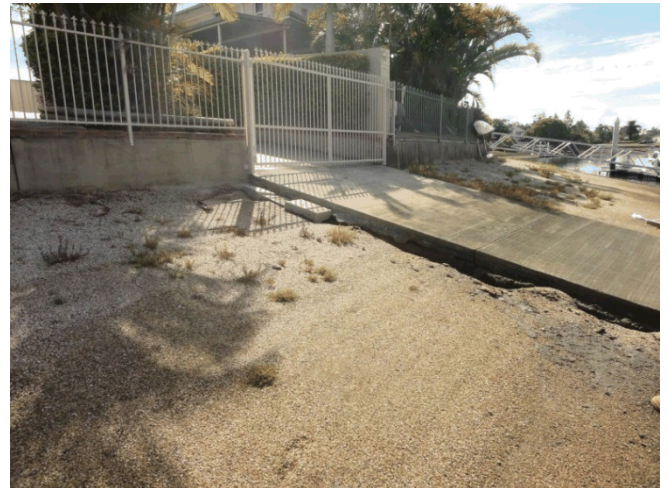
Example: Ramp erosion - owner responsibility
