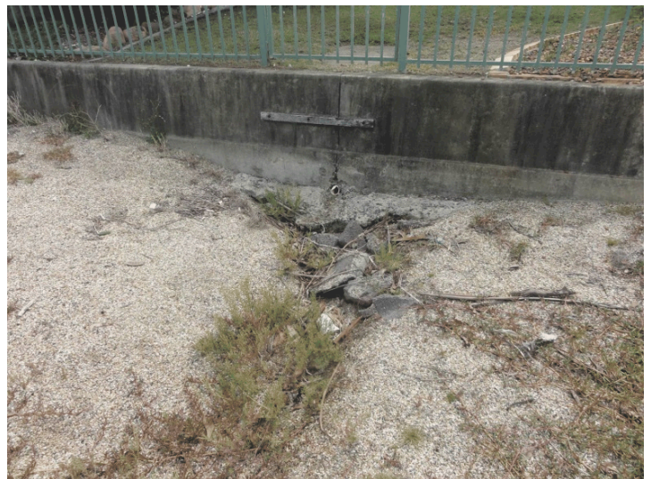
Example: Erosion - Condition State 4
