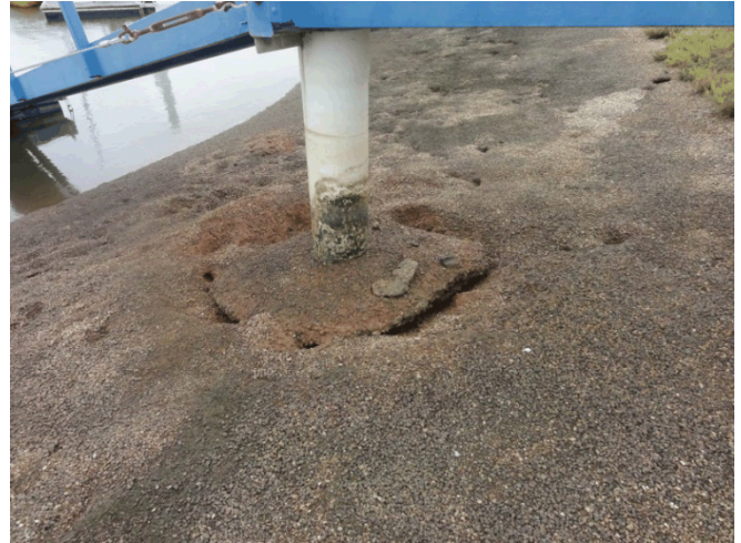
Example: Pile erosion - owner responsibility
