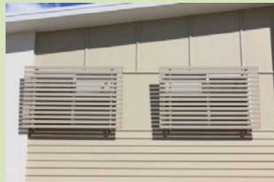
(Maroochydore) Fixed screening over windows is not a desirable solution to overlooking as shown above. Windows should be offset or have an appropriate separation distance.
