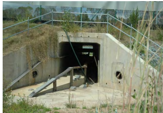
Engineered green infrastructure Koala Movement Underpass, SEQ
