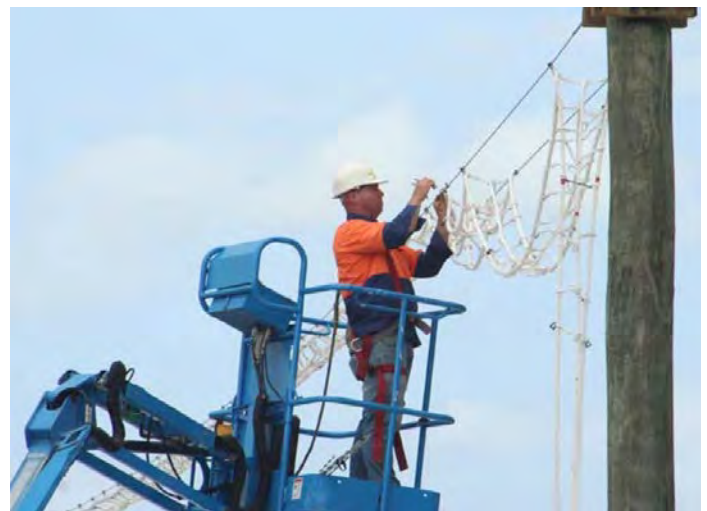
Rope bridges connect habitats and enable climbing fauna to cross roads, railway lines and easements safely (NSW).
