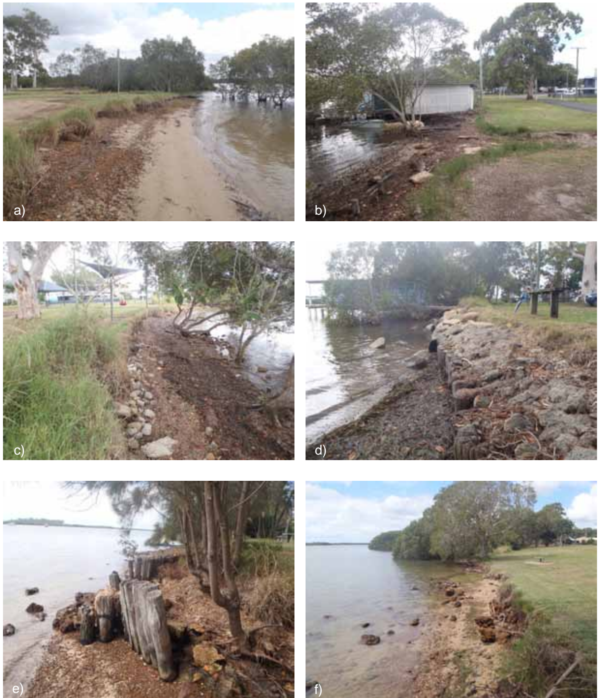
Figure 7-2 Example Shoreline Condition throughout Donnybrook Study Area: a) Sandy Shore with Erosion Scarp; b) Boat Shed; c) Loose Rock and Mangrove; d) Deteriorating Rock, Concrete and Timber; e) Deteriorating Rock and Timber; f) Loose Rock and Erosion Scarp
