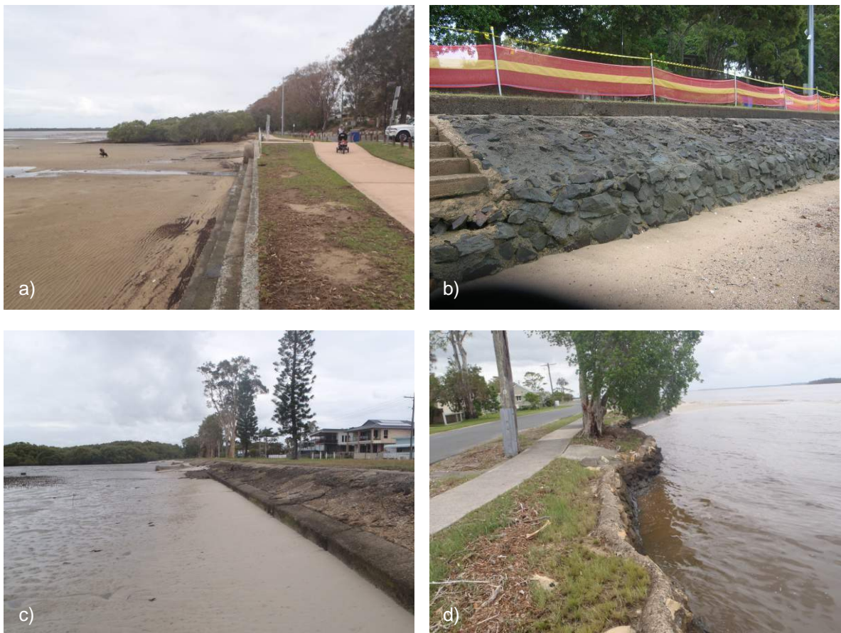
Figure 3-3 Examples of Revetment Seawalls throughout the Northern Bay SEMP Study Area: a) Stepped Concrete, Deception Bay; b) Stone Pitched, Deception Bay; c) Slopped Concrete, Godwin Beach; d) Rock and Concrete, Toorbul.
