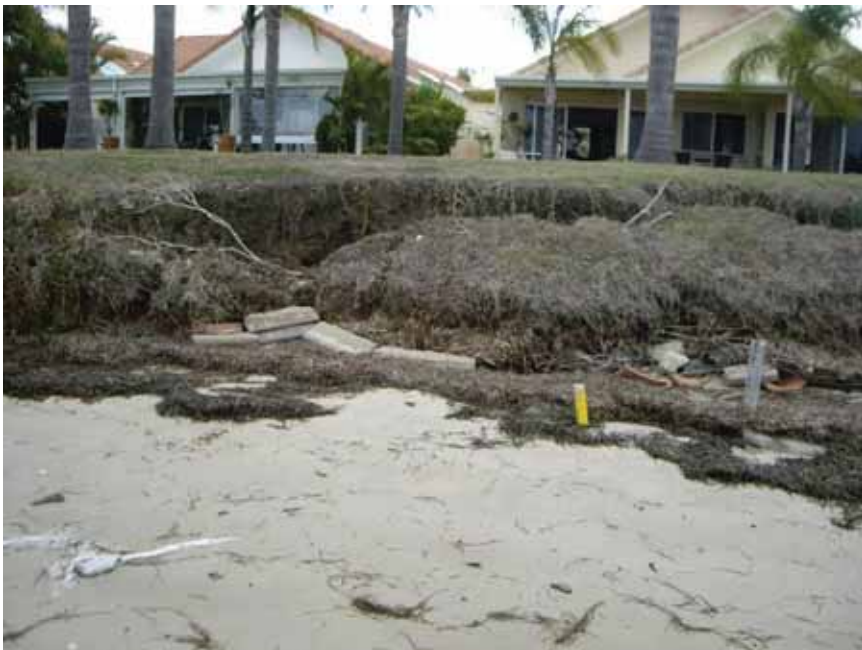
Photo Plate 9-2 Erosion south of marina
