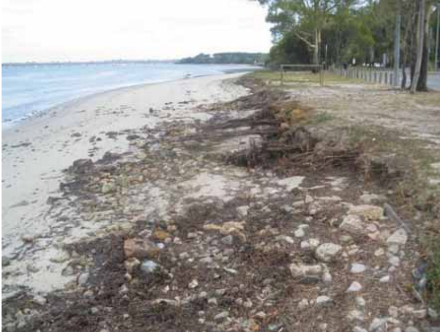
Photo Plate 9-5 Minor erosion south of boat ramp
