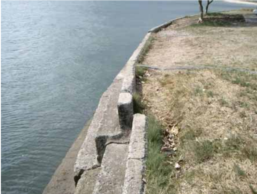
Photo Plate 4-5 Seawall movement north of Shirley Creek
