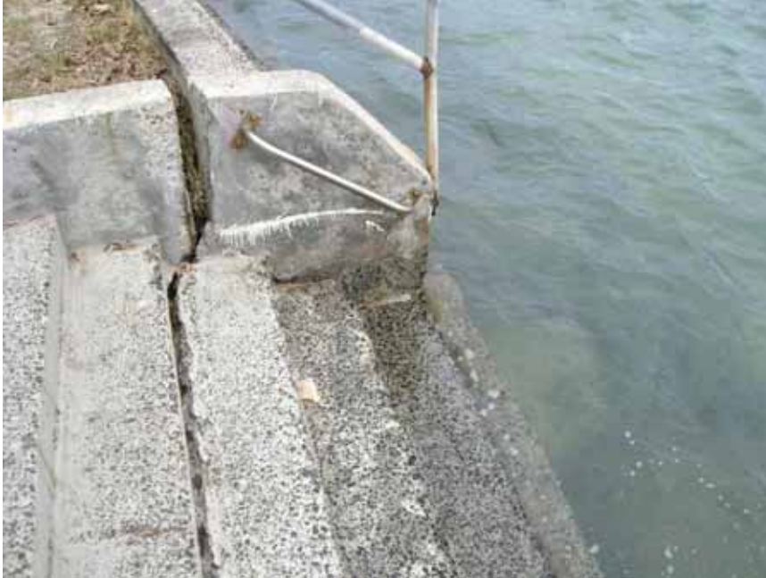
Photo Plate 5-7 Undermined sea wall and stairs north of bridge
