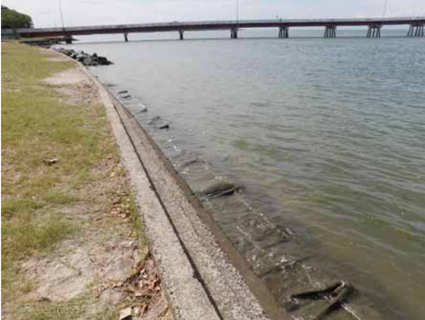
Photo Plate 5-5 Sea wall and sandbags north of bridge
