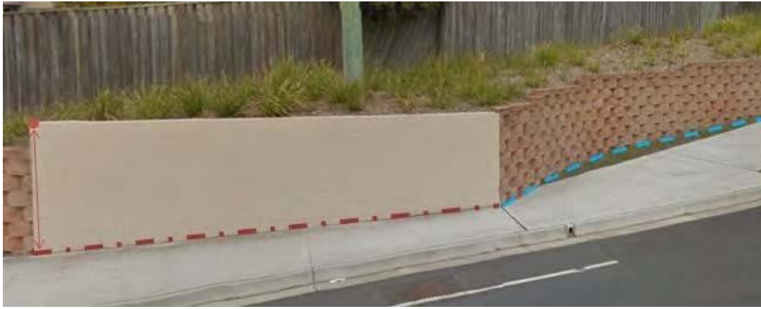
Figure 22: Retaining walls are captured at the base of the wall where it intersects with the ground (red) and the height is taken from the highest point. Features should be split where there is a material or construction method change (blue).
