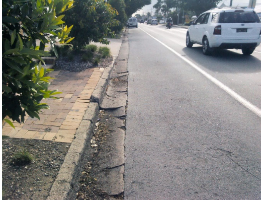
Figure 31 - Example of kerb and channel defect (Anzac Ave, Kallangur)
