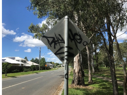
Figure 32 - Example of signage defect (Todds Rd, Lawton)
