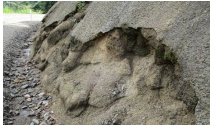
Figure 7 - An example of a condition 4 rated retaining wall in need of rectification or renewal. This eroded anchored wall on Goat Track Road will be renewed in FY2022
