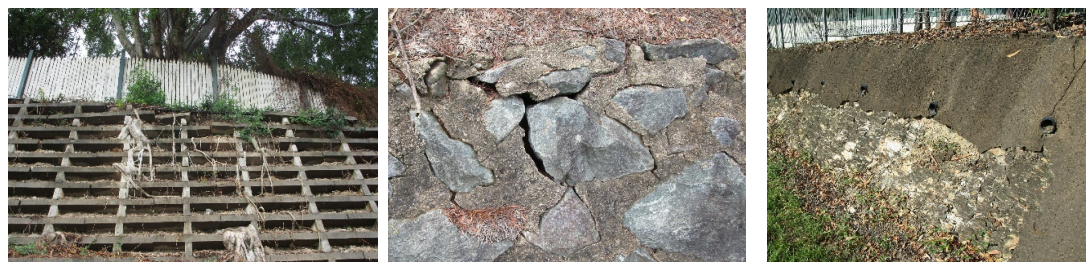
Figure 28 - Examples of retaining wall defects including (from left to right) vegetation damage on Albany Forest Drive crib wall, cracking of wall front, and erosion of sprayed concrete wall both on Old Northern Road.
