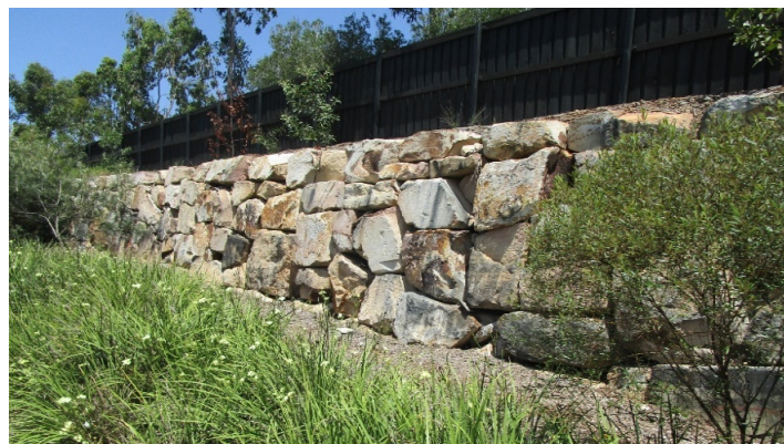
Figure 16 - A rock constructed retaining wall in the land improvement category at Mapleton Drive, North Lakes.
